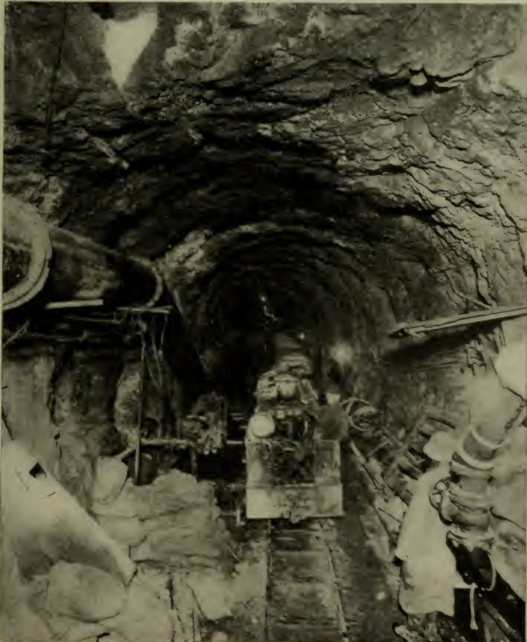
Section of uncompleted Tunnel, showing Pipe for Delivery of Compressed Air on Left. NEW WATER TUNNEL AT CHICAGO.
